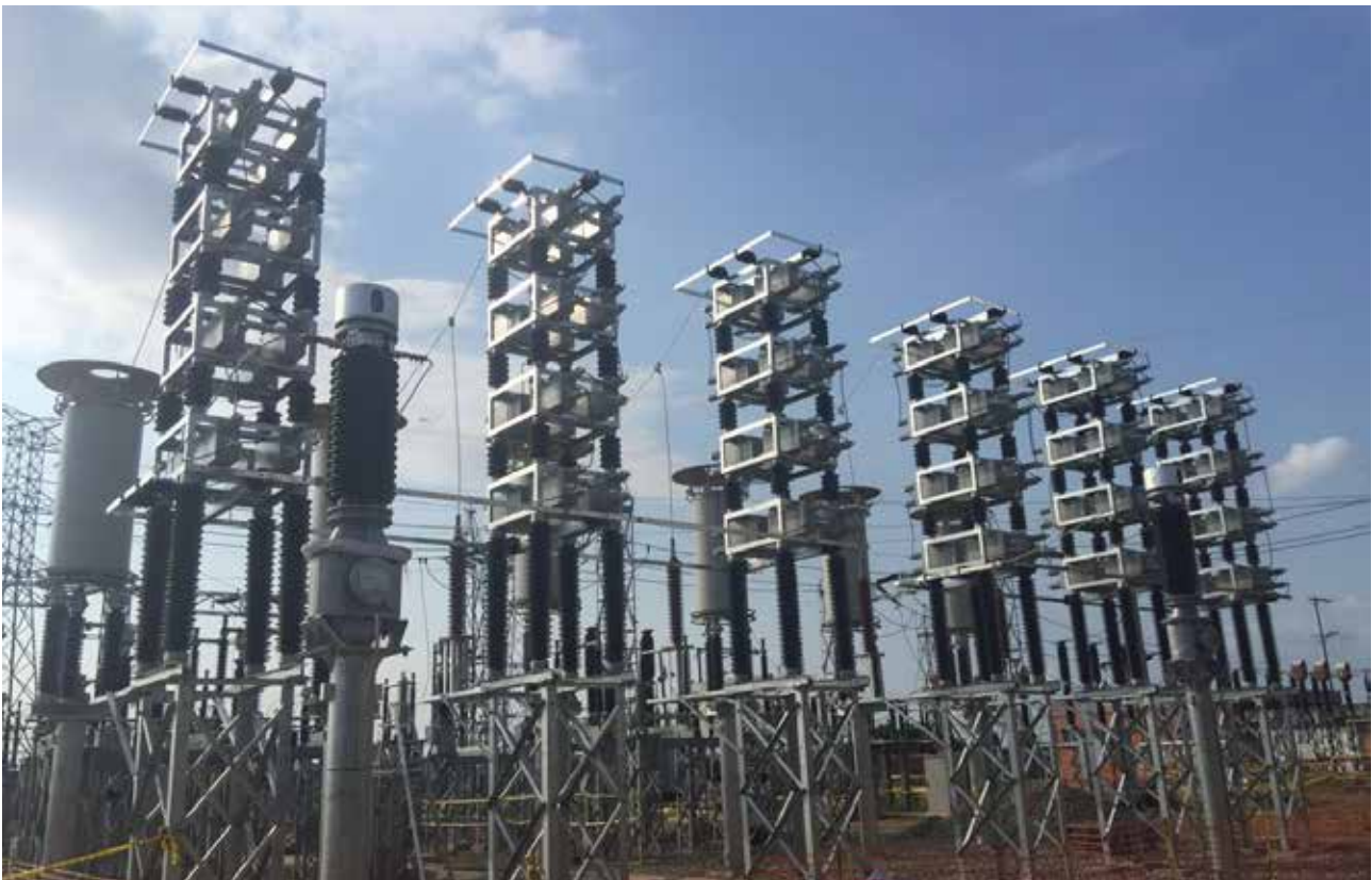
115kV shunt capacitor installation in Colombia
