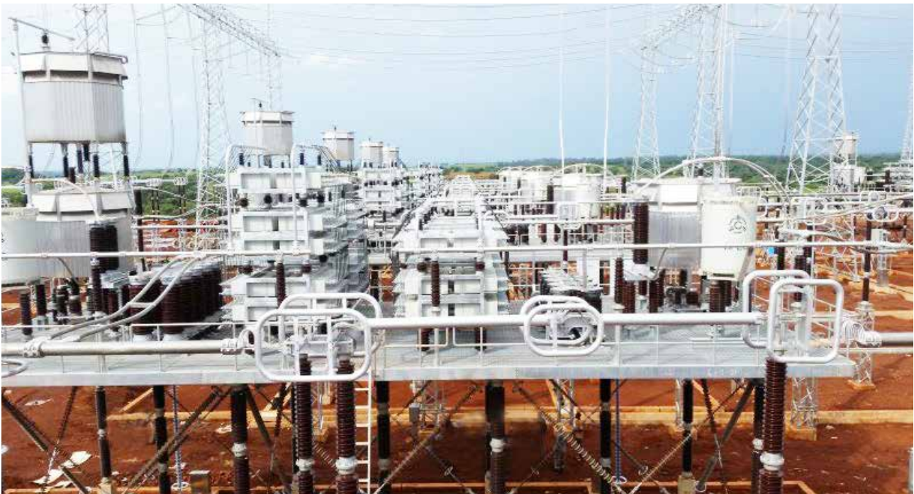
500kV series capacitor bank in Ethiopia
