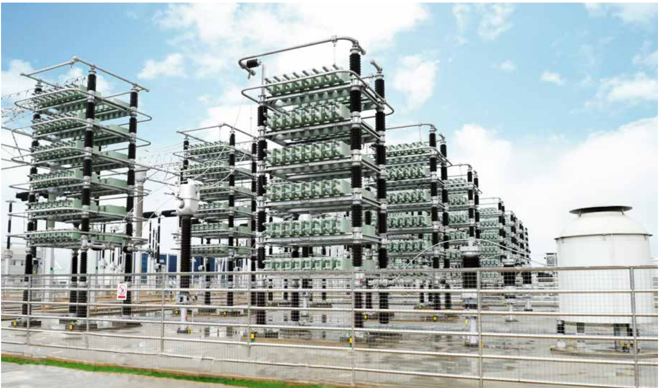
500kV shunt capacitor bank at Suidong convert station in China
